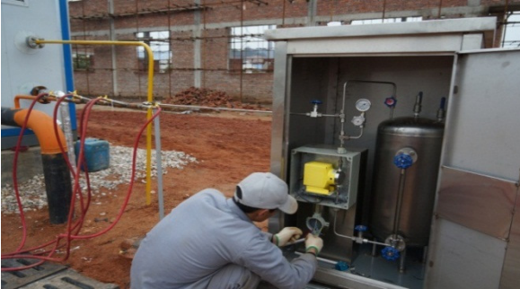
Figure 1: An on-site technician is checking the pressure regulator.
